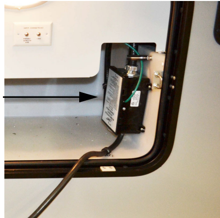
Automatic Power Transfer Box (Located inside water service center compartment) -Typical installation shown
