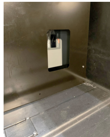
Inverter Unit (Located inside a right side outside storage compartment) -Typical View
