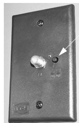
TV Signal Amplifier Power Switch (Located in an overhead cabinet or mounted on a wall near the TV) -Typical View
