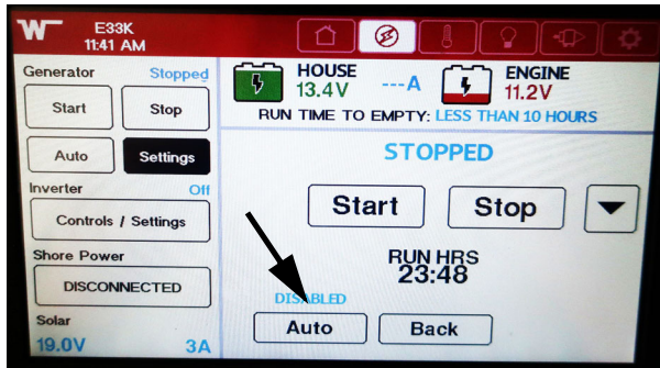
The Auto Operation Condition is displayed as Enabled, Disabled, or Locked out. -Typical View
