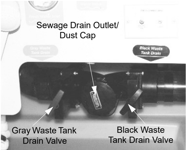
Holding Tank Drain Valves (Located in water service center) -Typical View Black and Gray Waste Tank Drain Valve positions may be reversed, depending on floorplan and tank location.
