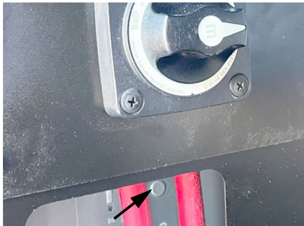
Ensure that the inverter box power button is pushed in for the monitor panel to be able to operate the inverter. -Typical View
