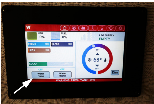
“Home” Screen • Tap Water Pump to turn off/on -Typical View
