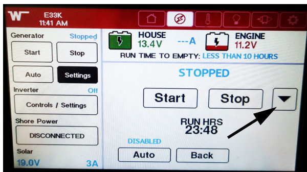
Select the down arrow to view the next screen. -Typical View
