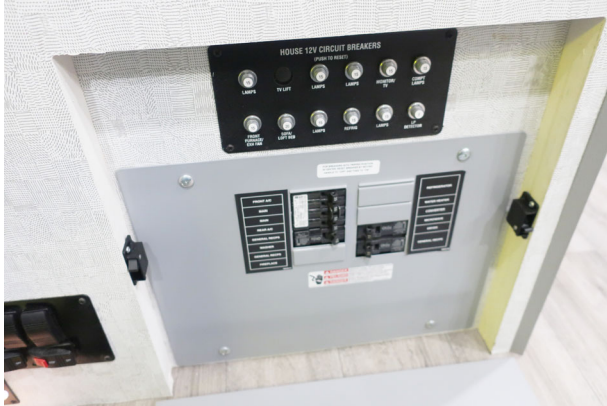
House 12-Volt Circuit Breakers -Typical View
